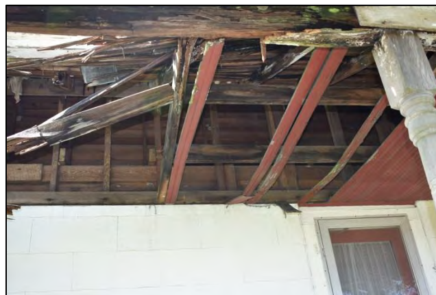
Figure 19: View to second floor of house through dilapidated porch roof
